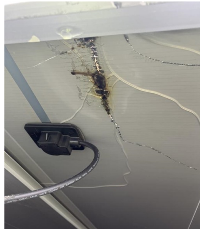
Module crack ground fault
