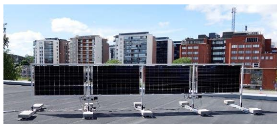
Figure 2: Vertical bifacial array in Turku, Finland.
