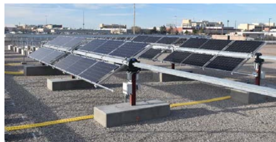
Figure 4: Single axis tracker with bifacial module strings in New Mexico.
