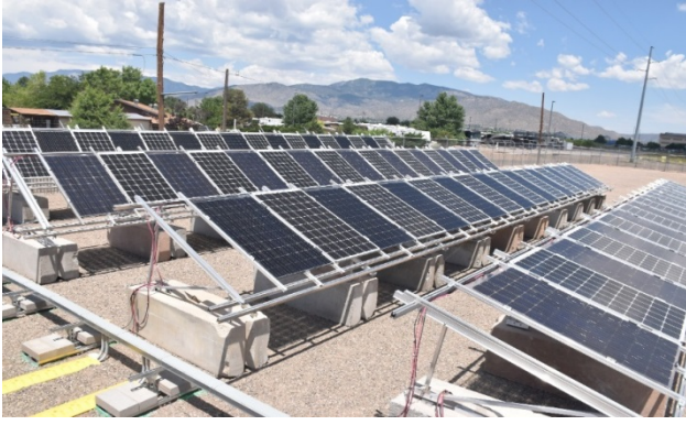
Fig. 5. Bifacial PV module test bed at Sandia. Four rows of PV modules with tilt angles from 15^\circ to 45^\circ . Backside irradiance measured for top and bottom of PV module near the center of each row. Front side irradiances are also measured.
