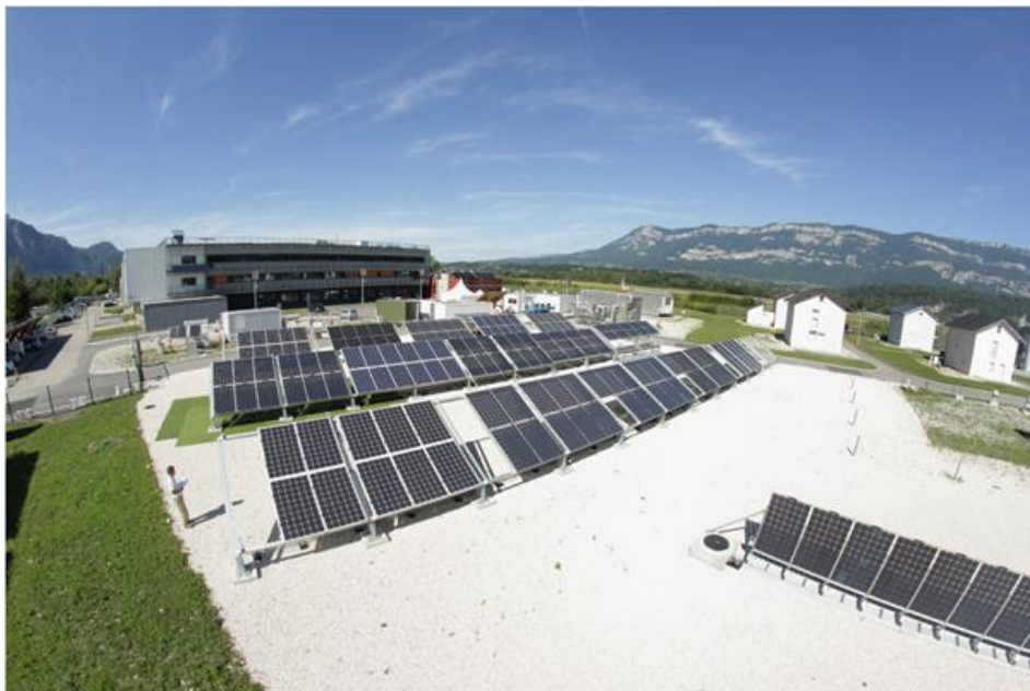
Figure 69: View of INES bifacial PV field test site.
