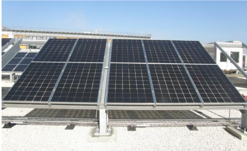
Figure 70: Front view of PV bifacial modules under test at INES site.
