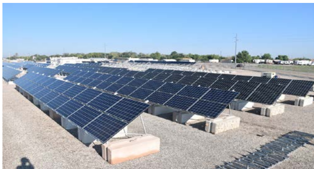
Fig. 2. Canadian Solar Modules at Sandia National Laboratories in New Mexico.
