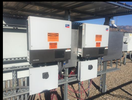
Inverter MPP Data Collection
