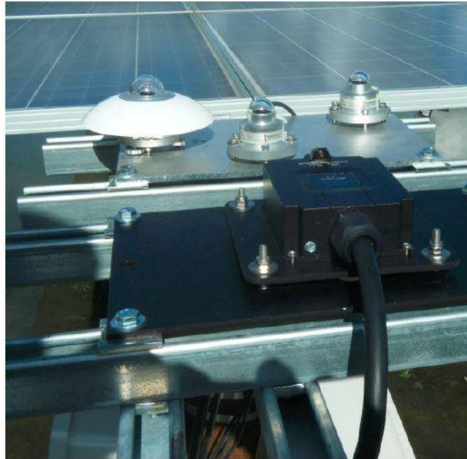
Fig. 1. Monitoring Station with SR20 (Left), LP02-1 (center), LP02-2 (right), self-cleaning reference cell (foreground), and reference module (back right)
