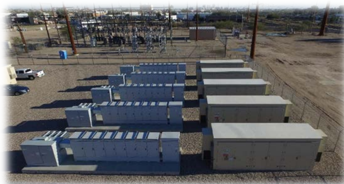
Next Era's Pima Energy Storage System (PESS)
