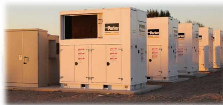
EC&R's Iron Horse Energy Storage System
