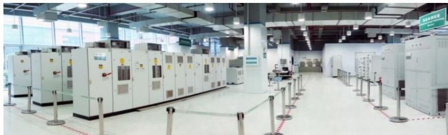
Labs with 1.5MW PV simulator
