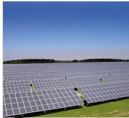
PV Power Plants
