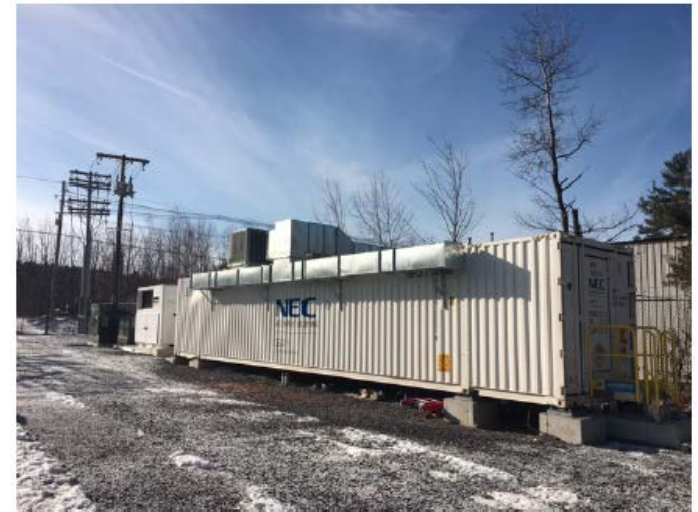
Sterling Municipal Light Department 2 MW, 3.9 MWh system
