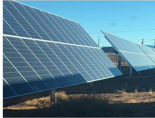
Row-to-row shading during BackTracking due to tracker error.
