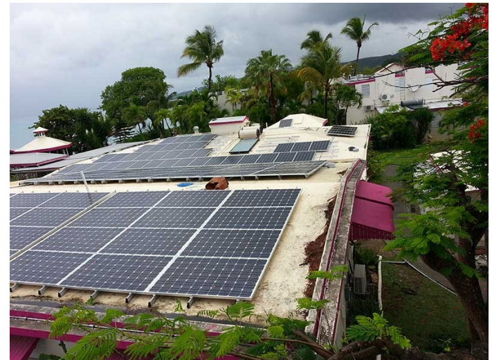
55kW rooftop PV on hotel in St. Croix
