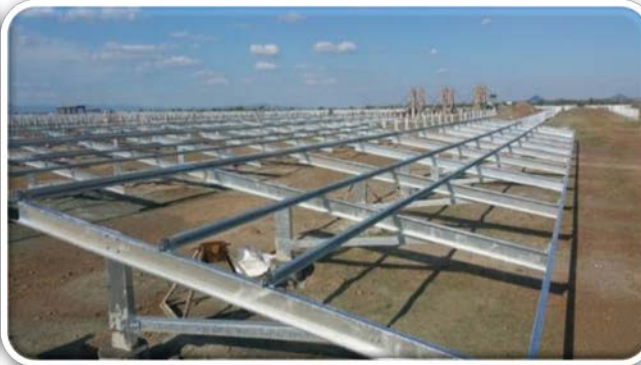
Place: India Time: 2017 Scale: 390MWp
