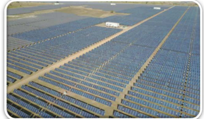
Place: India Time: 2016 Scale: 60MWp
