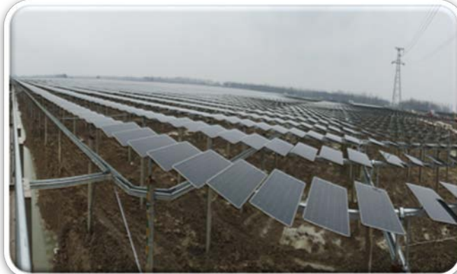
Place: Shou County, Anhui, China Time: 2016 Scale: 80MWp
