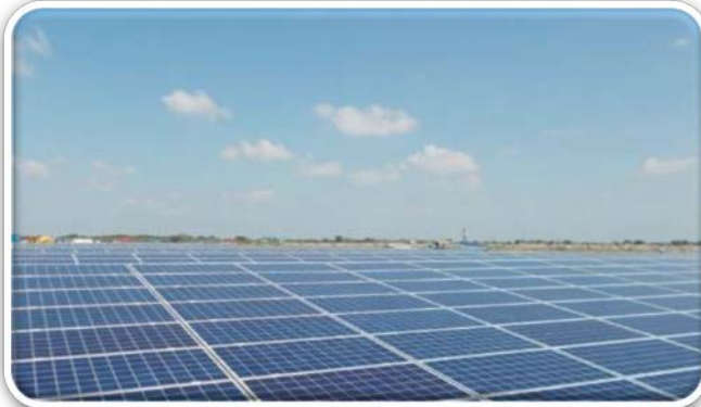
Place: India Time: 2015 Scale: 420MWp
