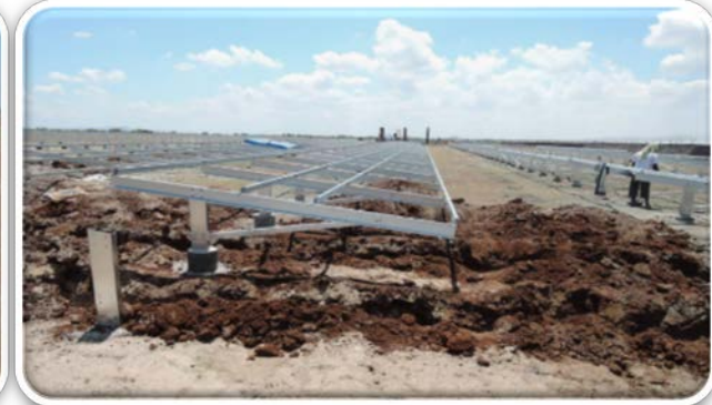
Place: India Time: 2015 Scale: 50MWp
