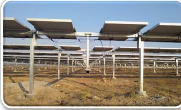
Place: India Time: 2017 Scale: 78MWp
