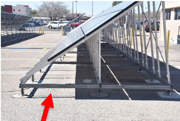
Lit ground beneath bottom module
