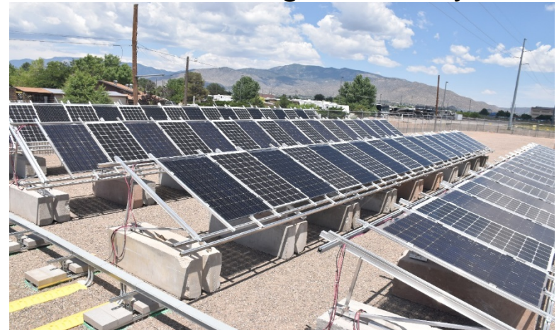
Fixed-tilt String-level Arrays
