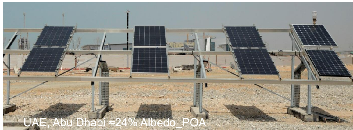
Albedo_POA: average albedo measured in tilt of module with silicon sensors.
