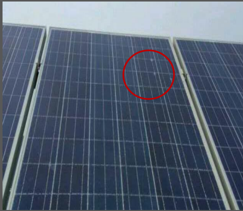
光伏板表面破损 (Gunshot Damage)
