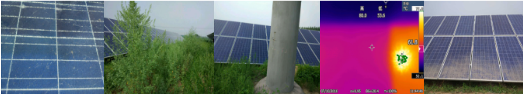
Glass (front-cover) breakage
