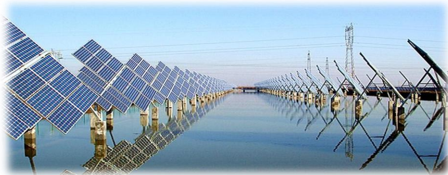
A distributed PV system installed in a fish pool, China.
