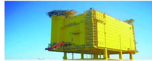
DolWin1 Converter Station
