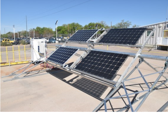
Fig. 2. Adjustable PV array at Sandia's Photovoltaic Systems Evaluation Laboratory.
