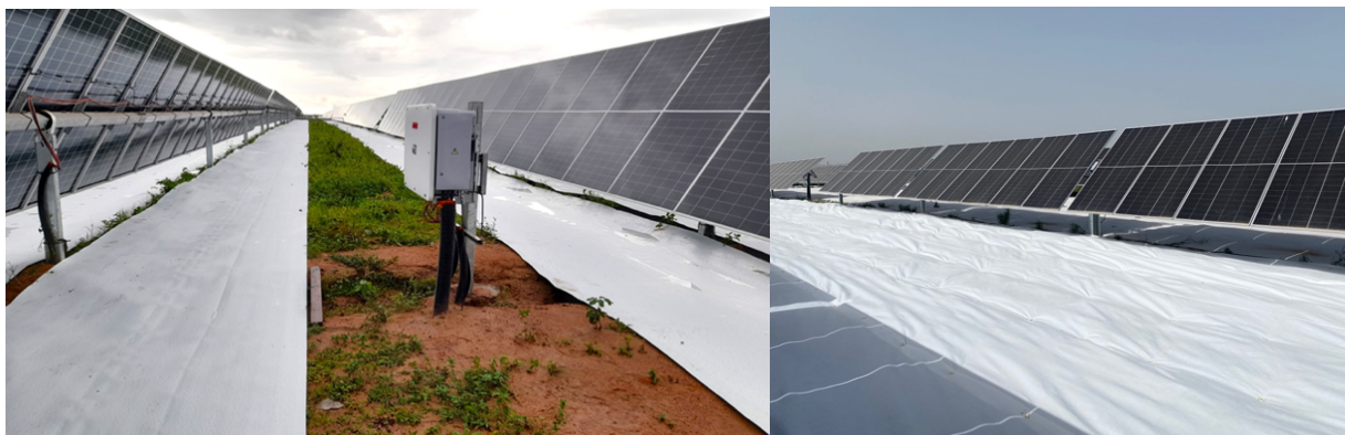
Figure 11 – Two examples for applications of albedo enhancers under bifacial trackers in large-scale PV power plants. Left: large-scale test of Solmax's Geolux albedo sheets (geomembranes) in Brazil (photo: Recurrent Energy), Right: Magnifield albedo enhancers (geotextiles) installed in a multi-MW power plant in Italy.
